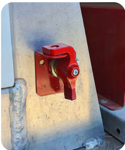
Battery Isolation Switch
